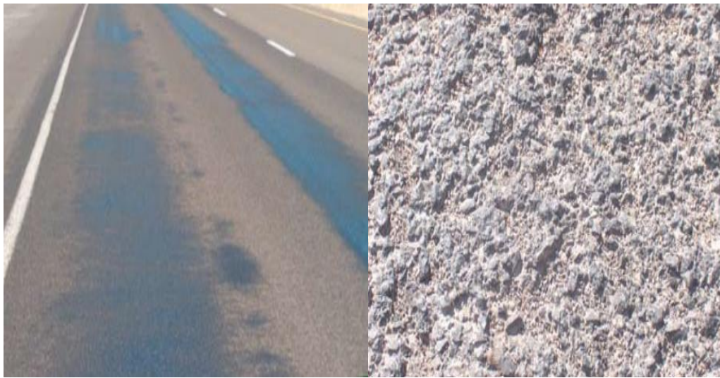
Figure 10. Slippage cracking & Weathering and raveling.
